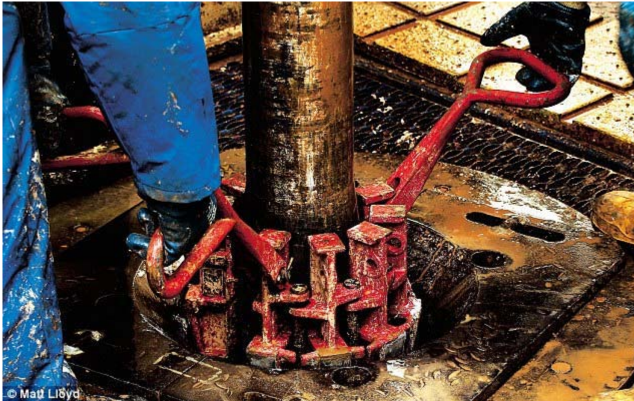
Drilling through more than 8,000ft of rock at a test-drilling site in Lancashire. It is no exaggeration to state that shale gas could transform the prospects for the entire British economy
